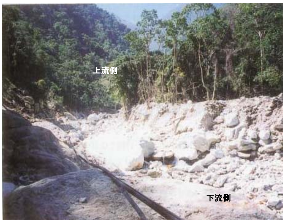
Photo 2 Eroded reach due to debris flow in the upstream of the fan head
